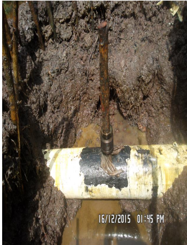
3" NIPPLE INSTALLED BY VANDALS
